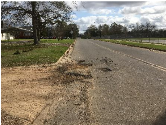
Figure 19. Potholes on East Palm Street. (Photo: Ariel Godwin)
