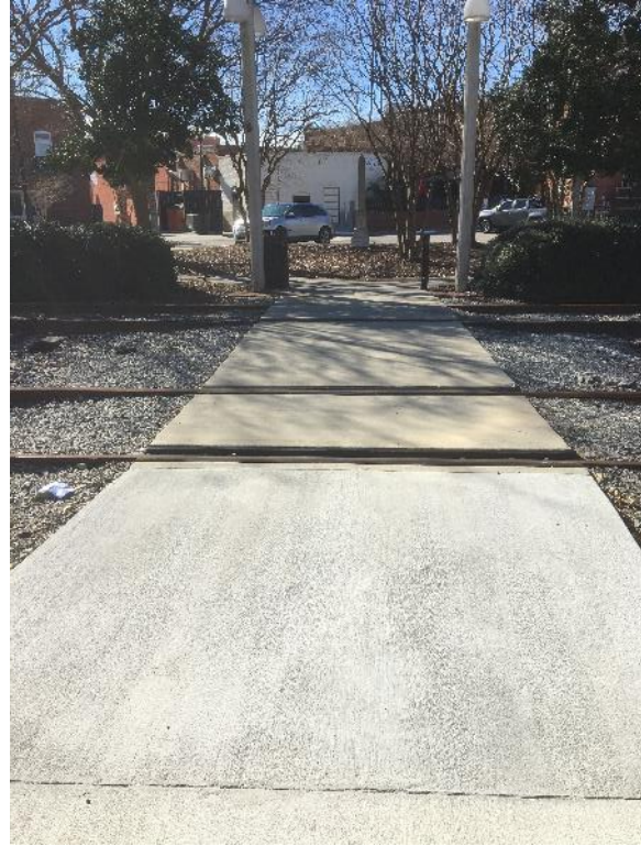
Figure 16. North-facing view of improved pedestrian railroad crossing in Tifton. (Photo: Ariel Godwin)
